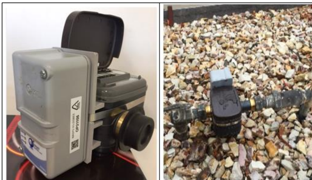
Figure 3. High resolution water meter and logger (left) and this installed (right)
